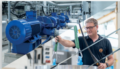
Pumps and compressors
