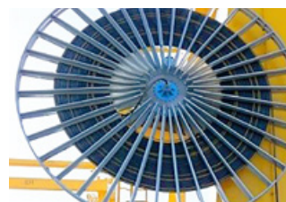
Unwinding and winding equipment
